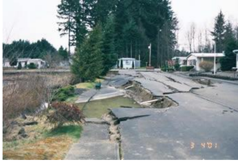
Figure 3.1-7 Example of Lateral Spreading. Lateral spreading Sunset Lake trailer park in Tumwater.
