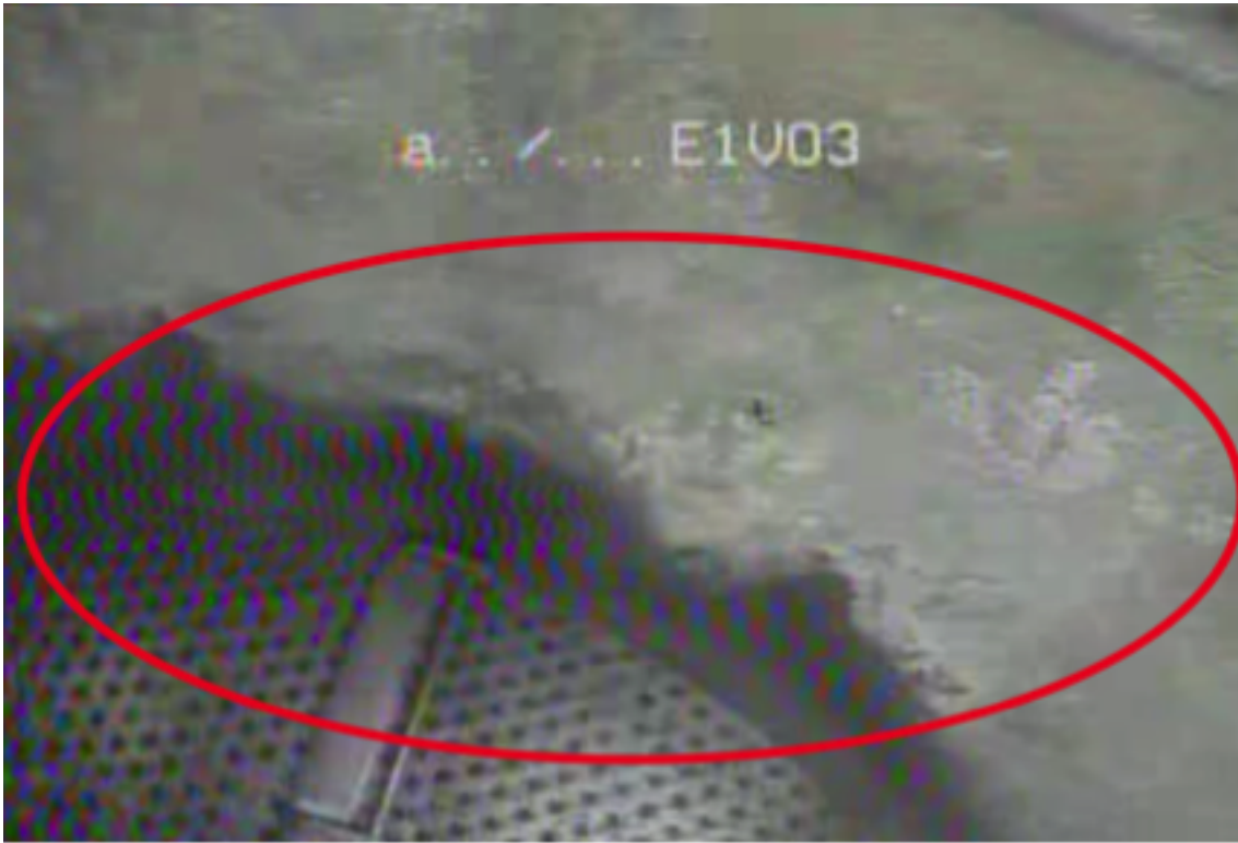
Figure 8.3: Steel jacket collapsing
