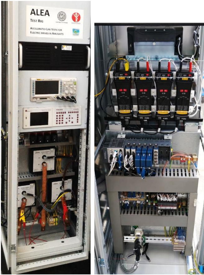
Fig. 13 Front view and internal view of the DAQ electrical cabinet.
