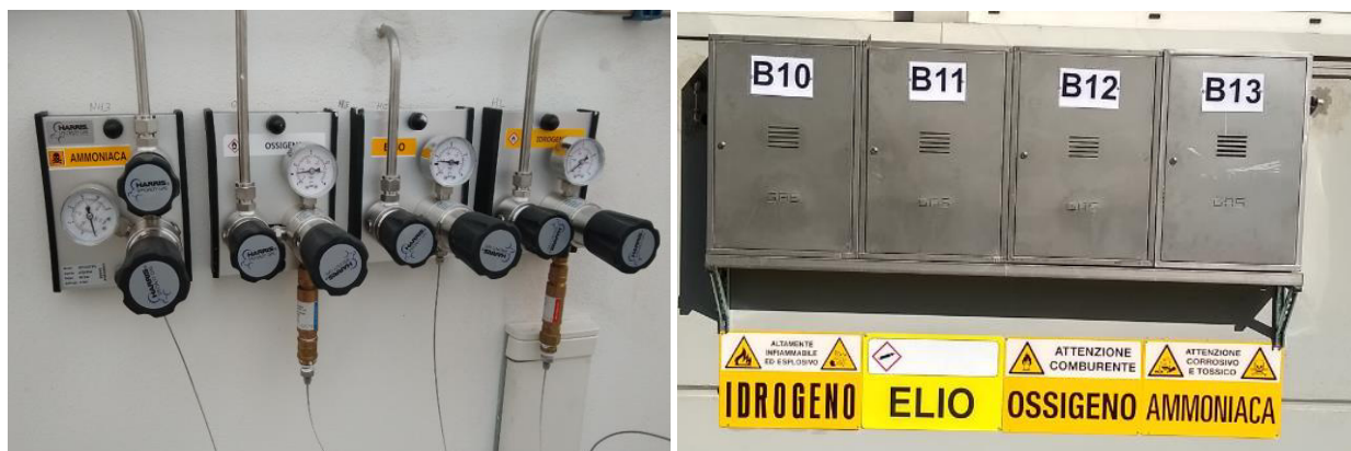
Figure 3.24: New gas supply lines for the QCELL system: on the left, the indoor second stage gas pressure regulators; on the right, the outdoor gas cabinet. Labels are in Italian because the lab sites belong to an Italian institution.
