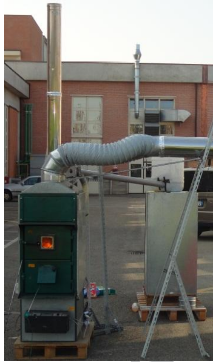
Figure 3. Pellet combustion facility
