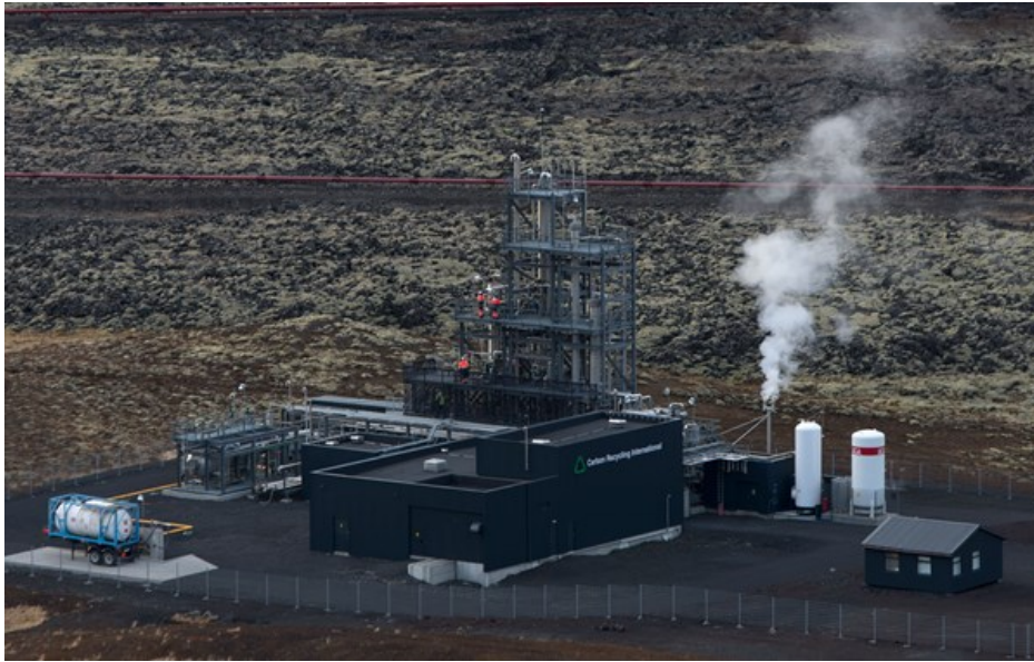
Methanol plant at Svartsengi, Reykjanes for Carbon Recycling International
